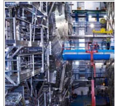
Installing the beam pipe at the LHC on 16 June: the final section of 1
